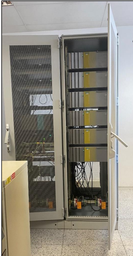
Server SIMENS SIMATIC
