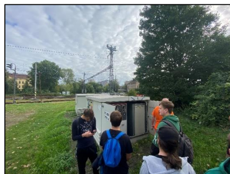
Bloková transformovna TČD 1100 3AC 50 Hz 22kV/IT
